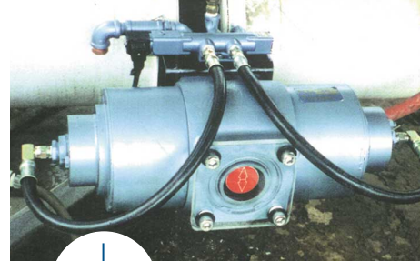
AIR SEPARATION PLANT ACTUATORS
