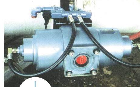
AIR SEPARATION PLANT ACTUATORS
